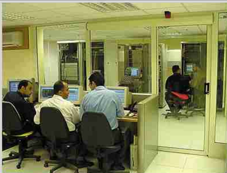
Raya Telecom created a fully automated network operating center, equipped with the latest security measures, and complemented its services with a state-of-the-art data center.
